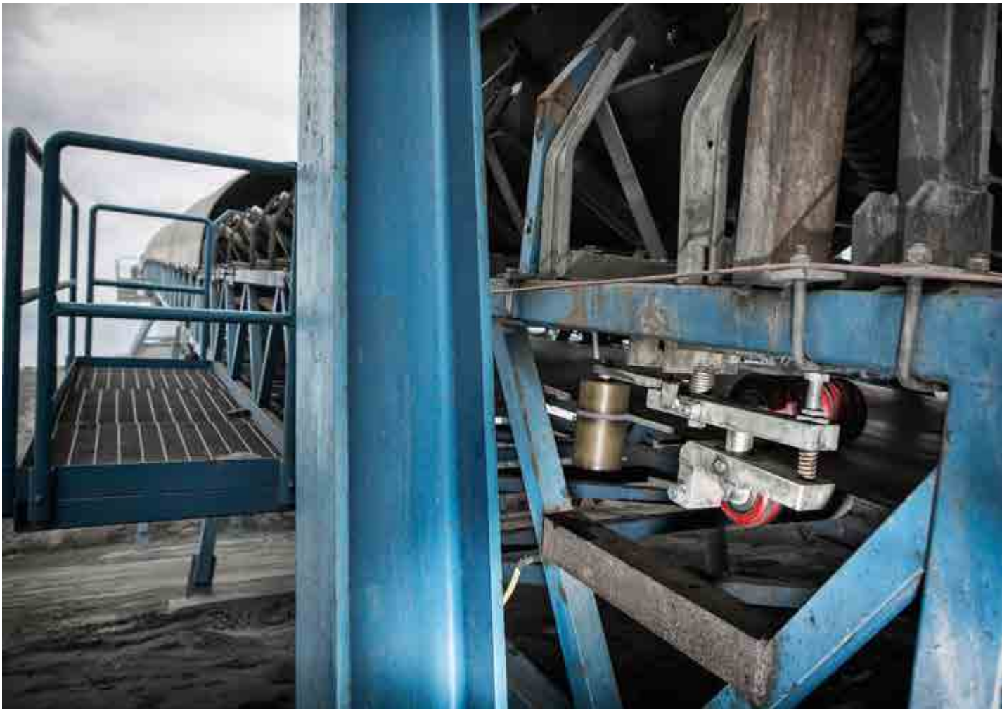
Inline Tracker in operating environment
